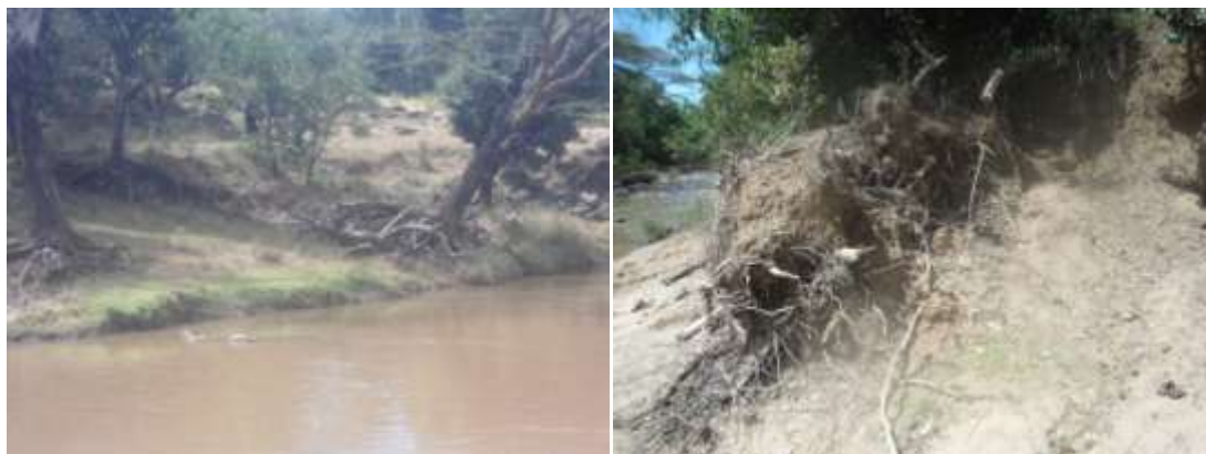
Figure 3.3: River banks of lower Nyangores River where trees have exposed roots caused by washing away of the poor cohesive sandy soil.
